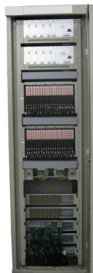
IP-enabled information transmitter Telemetering and controlling equipment
